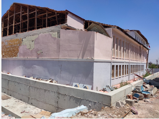
Damage to Roof truss
